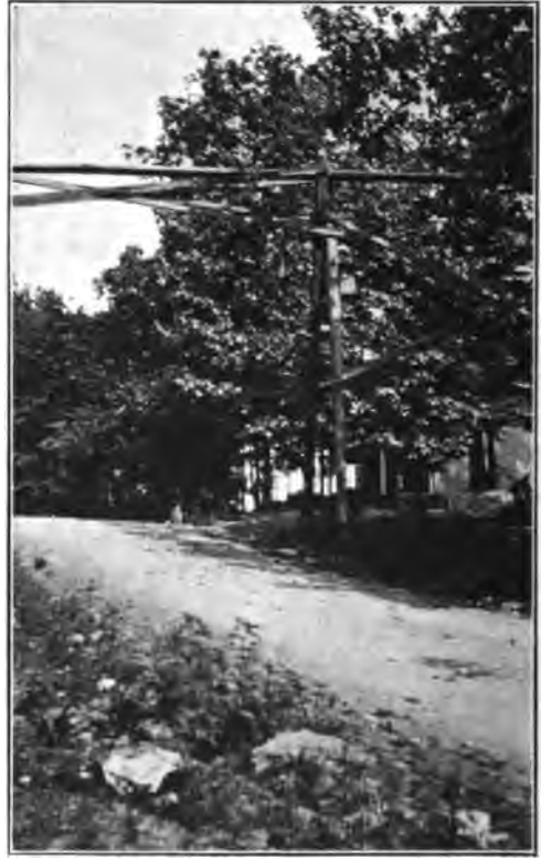
FIG. 7. AIR PIPE CROSSING HIGHWAY.
