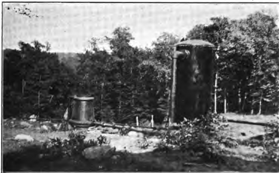
FIG. 8. RECEIVER AND REHEATER.
